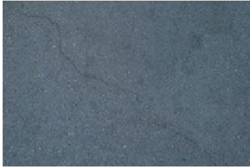
Fig. 3. Cracks in concrete building components
