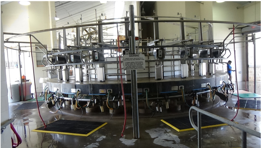
Fig. 2. Example of a collected image for the milking machine project.
