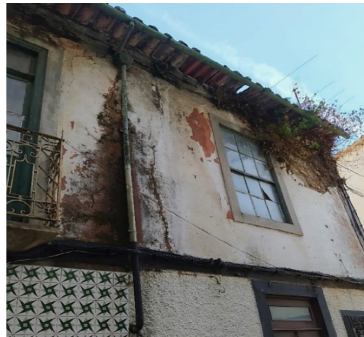
Fig. 6. Vegetation and algae in building façade.
