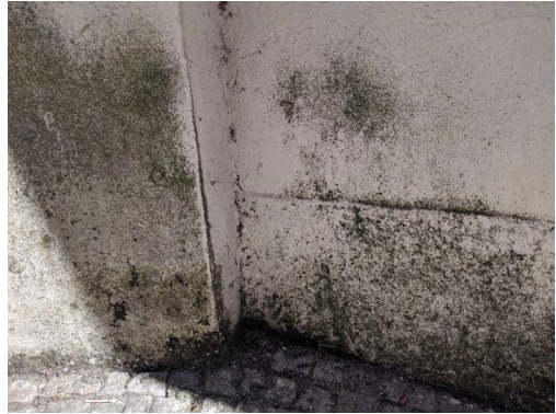
b) Detail of fungi in the façade
