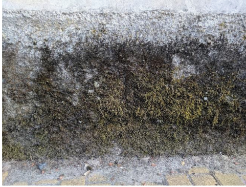
Fig. 2. Detail of a building façade with mosses.
