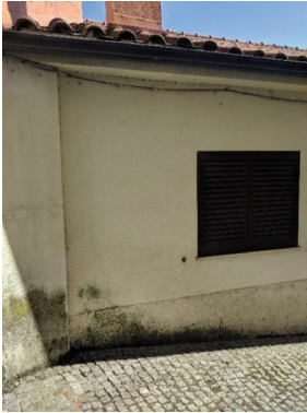
a) Façade with the presence of BG
