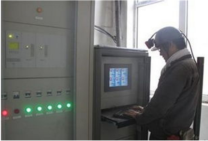
Fig. 2. On line monitoring system of transformer insulation fault
