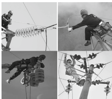
Fig. 2. Example of the action monitoring video image of the electric power maintenance personnel
