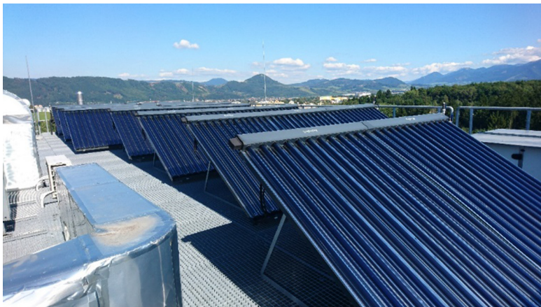
Fig. 4. Panels of solar system on the roof of building.
