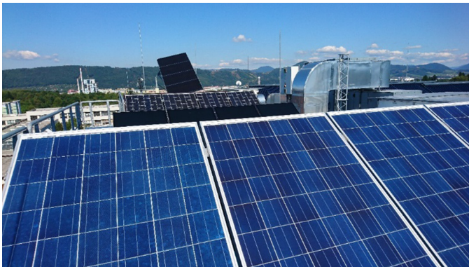
Fig. 1. Photovoltaic system on of the building. Last panel tracks the Sun
