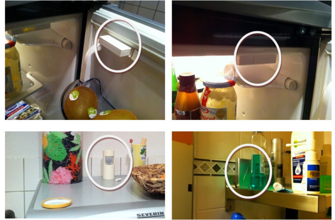
Figure 5. Examples of Home Automation Sensors Installed in the Test Households
