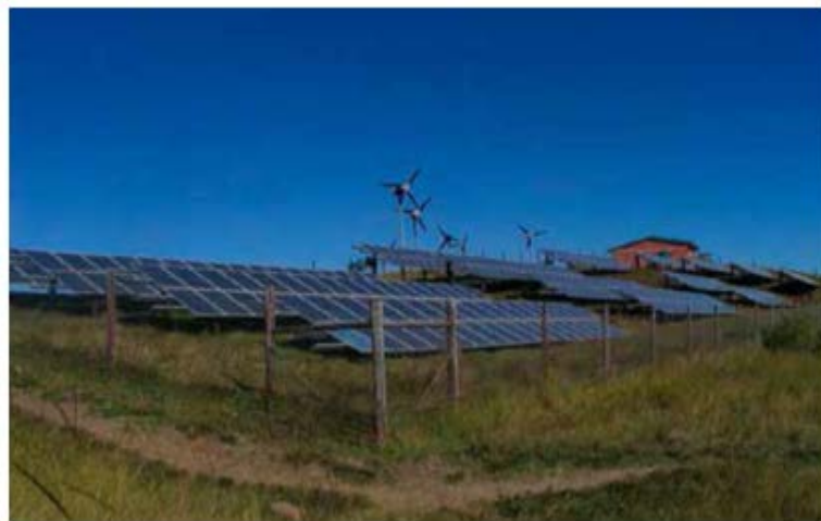
Fig. 2. Hybrid solar-wind mini-grid at Lucingweni Village in the Eastern Cape Province of South Africa
