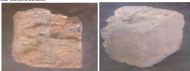
Fig. 6. Common Farm Brick collected from site shows weak bearing capacity and would crumble easily.
