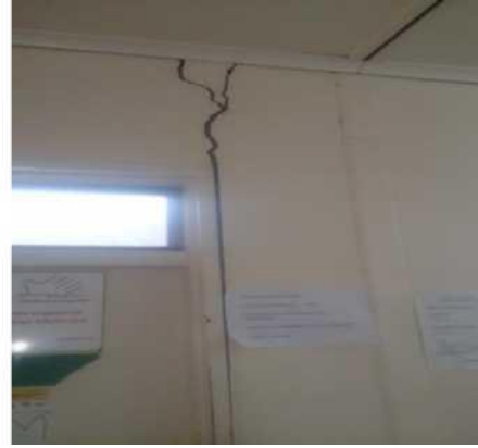
Fig. 3. Vertical crack on another building
