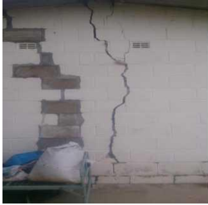
Fig. 2. A jagged vertical crack on the wall of a building
