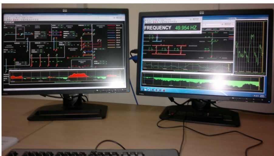
Fig. 3. Operator Workstation of the SAPP System Viewer (Source: SAPP, 2016).
